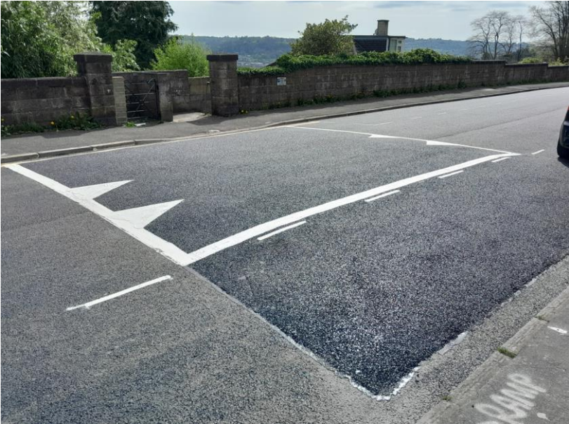
Example: Tarmac road humps and speed cushions are hard wearing and relatively low cost
